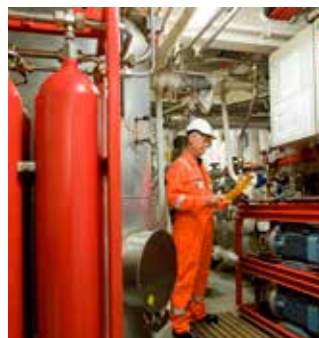
Fire safety equipment
